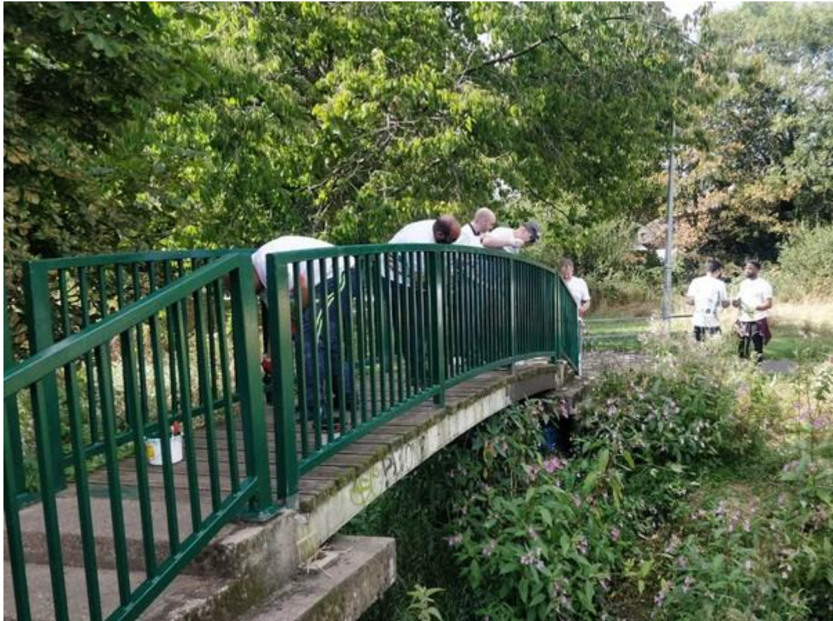
Photo caption: Staff from BNP Paribas painting the bridge at Green Lane Park
